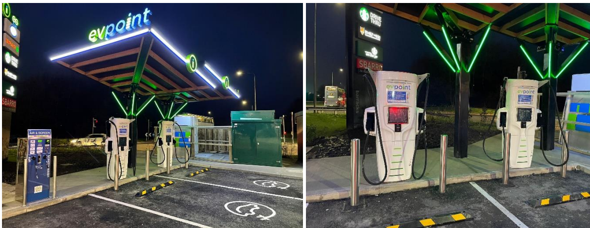
Photo of New 175Kw Ultra Rapid Chargers Installed at Euro Garage Petrol Station Barracks Road Burnley.
